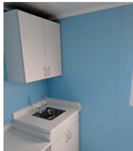
Hand wash sink with point of use water heater.
