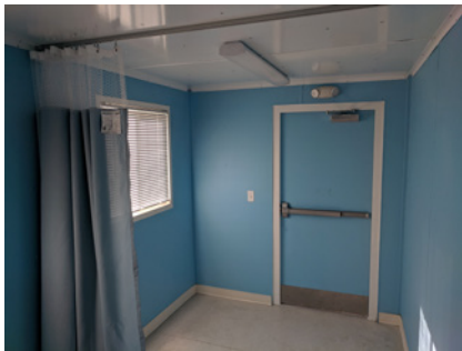
View from interior of exam room, looking toward entrance and waiting area. Push bar emergency exit device on door along with LED emergency lighting provides added safety.
